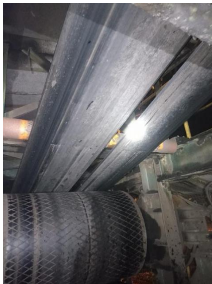
Gambar 2. Dokumentasi Kerusakan Belt Conveyor di Area C26 BoCT Sumber : Port Maintenance Bontang Coal Terminal, (2025)
